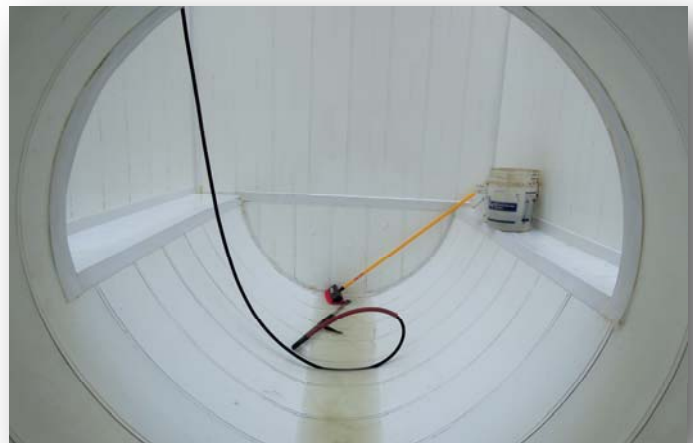
8' x 8' Junction Box with 84" Pipe lined with Danby PL3E PVC liner
