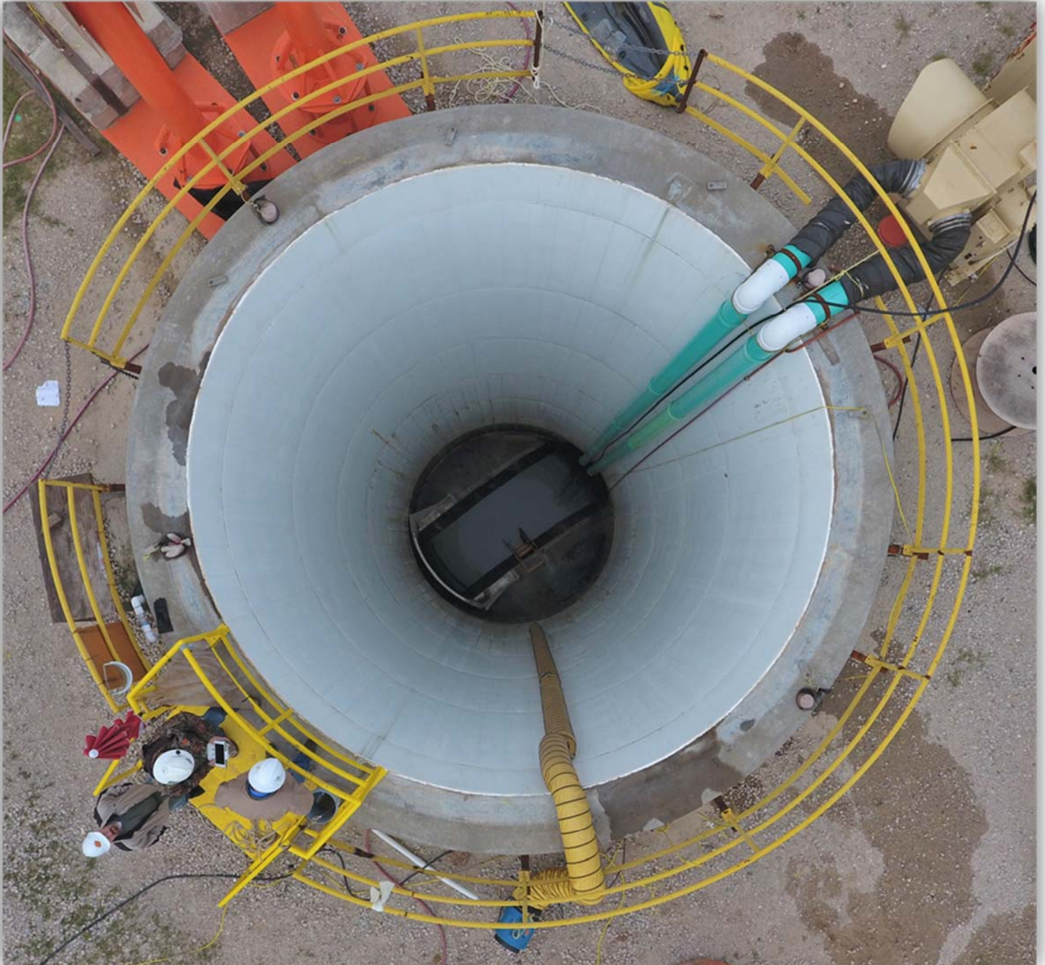
Structural Concrete Bypass Chamber – 20' diameter x 60' Depth over a 108" Sanitary Sewer Influent . Danby PL3E PVC liner installed during construction of chamber
