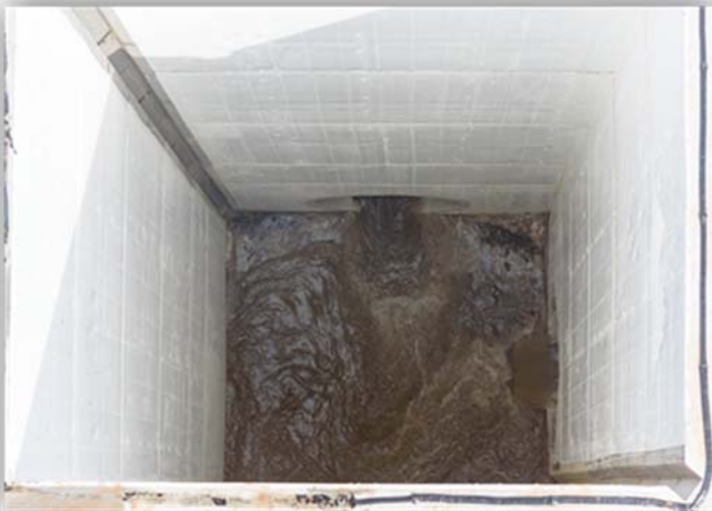
12' x 15' x 58' Depth Structural Concrete Diversion Junction Box lined with Danby PL3E PVC liner
